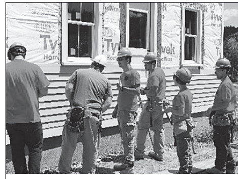
Penobscot Job Corps under instructor Luke LaChance install clapboard on the Fields House at Orrington.
