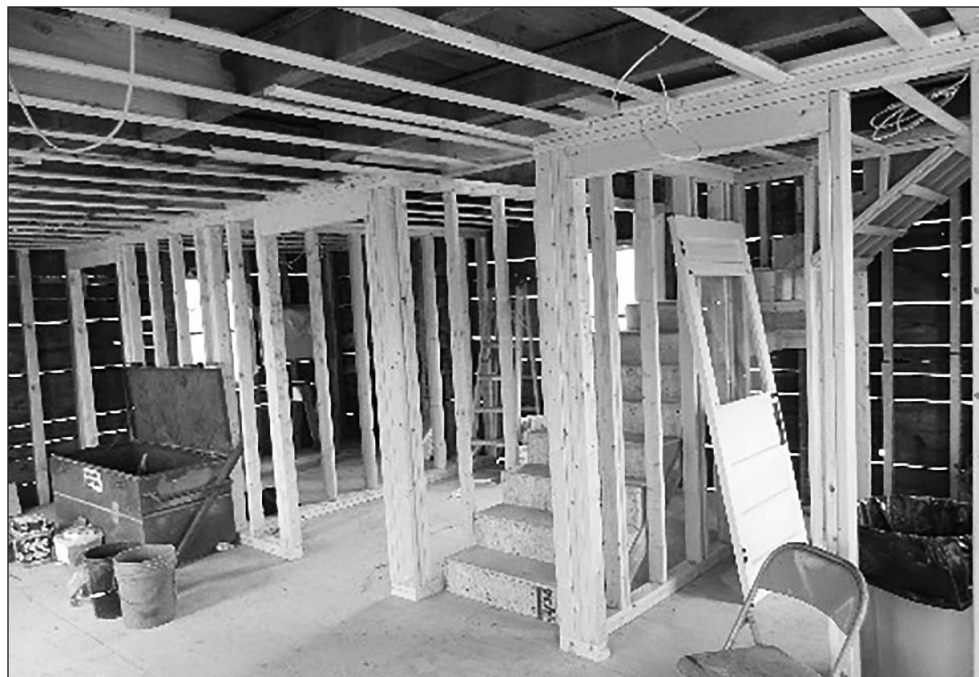
Interior framing and a new staircase in the Fields House are some of the projects completed by Job Corps.
