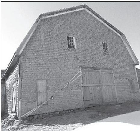
Back of the barn. We have issues with the piers and drainage around this area specifically.
