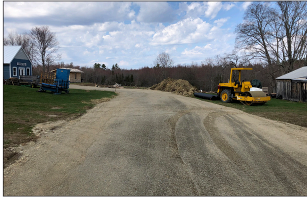
A road to the site of our relocated Carousel Building and our extended museum village.
