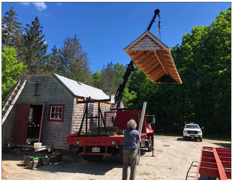
Temporary alteration of the Tom Flagg Smithy necessitated to meet height restrictions en route to Orrington.
