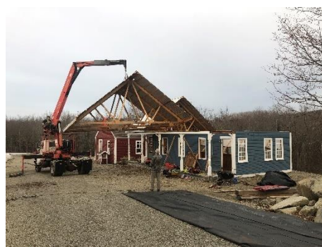
Doug Dolan & Cal McGraw seen here among the crew recently re-assembling buildings.
