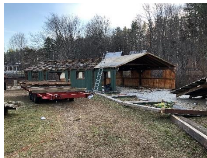
The future Car Culture Building ; the rebuild will include 20 more feet of space.
